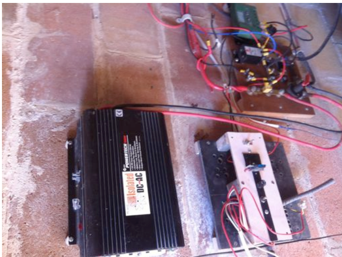
Barossa Club wind & solar power set-up.
